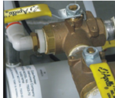
30 Gallon Tank Valves
