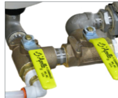
30 Gallon Tank Valves
