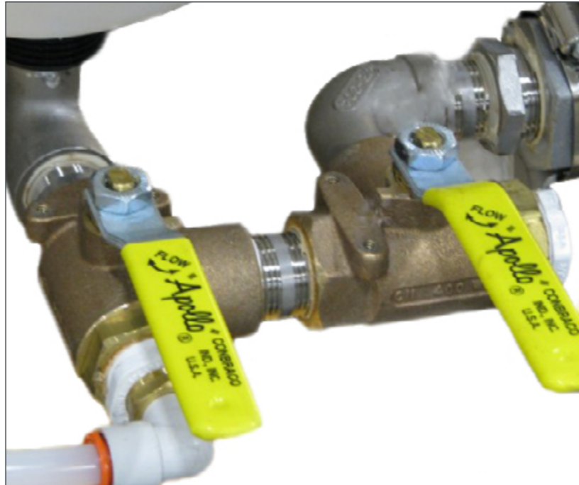
30 Gallon Tank Valves
