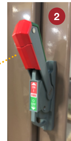
Control Panel Power Lever UP
